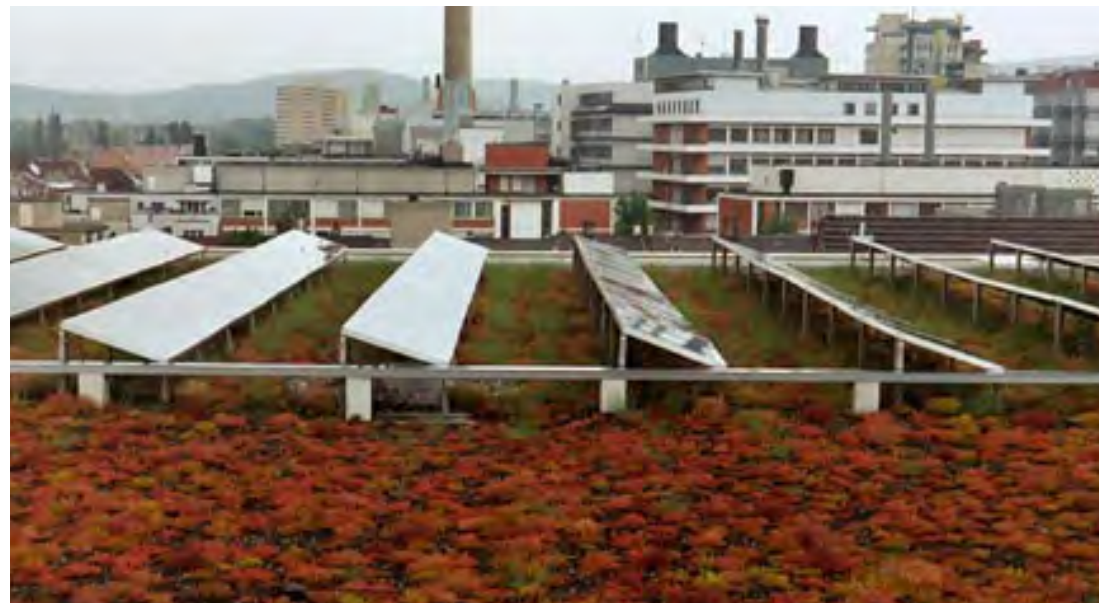
Figure 148: Biodiverse roofs with photo voltaic panels
