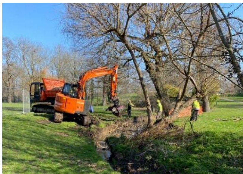
Figure 6-3 Removal of concrete to naturalise the existing riverbed Image Credit: 'Unblocking the Burnt Oak Brook Project' Report, Thames21
