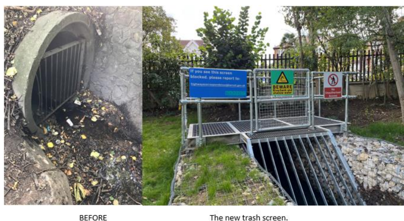
Figure 6-5 Before and after photographs of the trash screen at Friary Park
