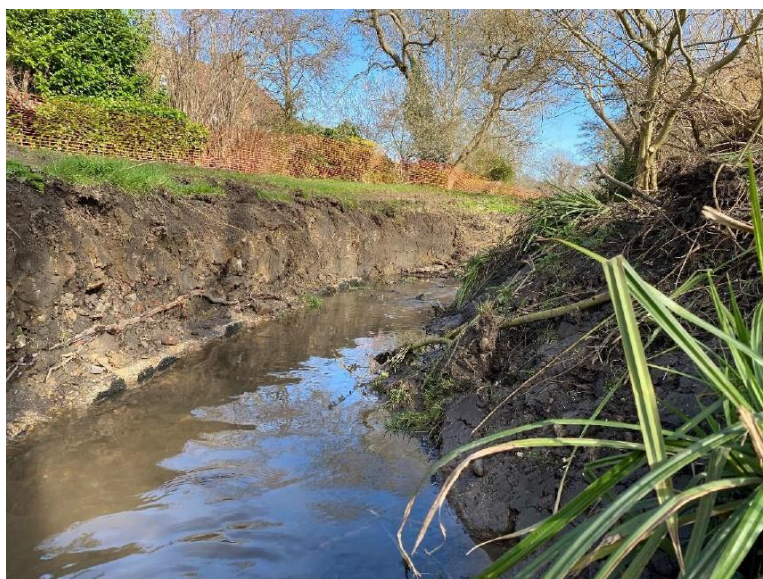
Figure 5-2 Riverbanks of the Burnt Oak Brook after concrete removal Image Credit: Unblocking the Burnt Oak Brook Project Report, Thames21
